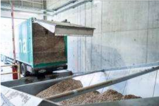
Image 1: The truck unloads wood chips, fresh from the forest, onto a drag chain discharger. The unloading process takes about 15 minutes.
