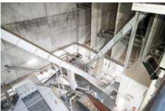
Image 3: Vecoplan supplied all the machinery for the plant and took responsibility for its assembly and commissioning.
