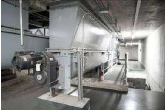
Image 4: Dosing screws gradually feed the fuel onto the conveyor system, which transports it into the feed hopper of the furnace.
